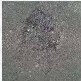
Asphalt showing scuffing
